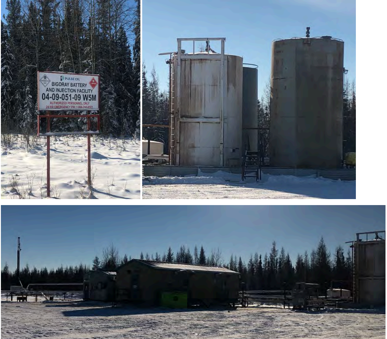
Figure 1: Bigoray Battery and Facilities
